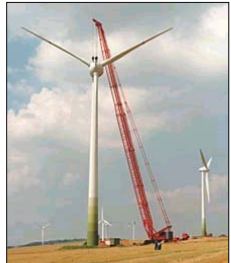
A Liebherr LR 1400/1 crawler crane lifts a 38 metric ton propeller 70 m for installation at a wind power plant in Dorntal, Germany. Normally two cranes lift and manipulate the propeller from horizontal to vertical, but in this case the task was accomplished with a single specially rigged crane. (Photo courtesy of Liebherr-Werks Ehingen GmbH.)
